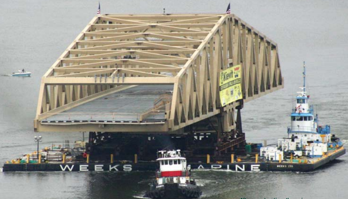
After construction, the swing span was floated down the Hudson on two welded-together barges powered by several tugs.
