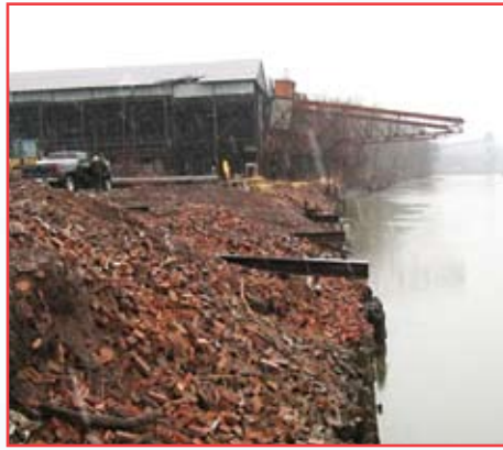
Cleaning up the debris from the old brickyard was quite a challenge. The lot had a lot of dilapidated buildings and even a landfill.
